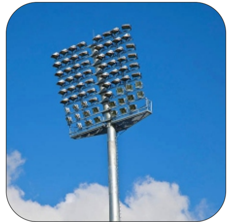
High Mast Light Pole
