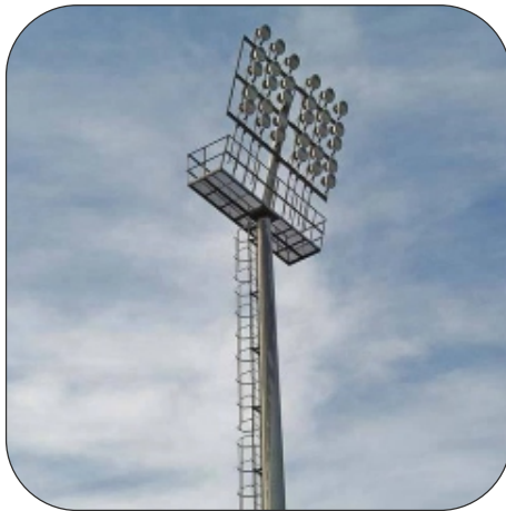
Stadium Mast Light Pole
