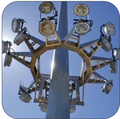
Mast Light Pole
