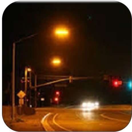
Low Pressure Sodium Street Lights
